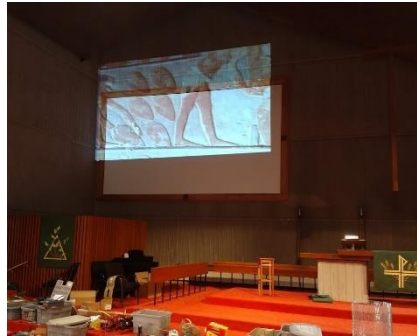
The new video screen is installed, and the projector image is being focused.
